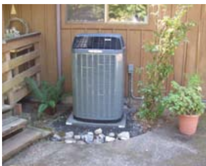
Trane High Efficiency Heat Pump Installed on an Existing home
