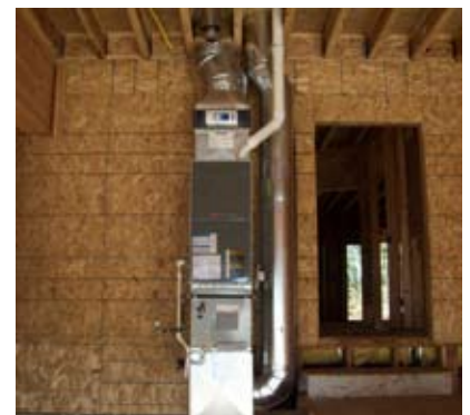
High Efficiency Gas Furnace and EAC
