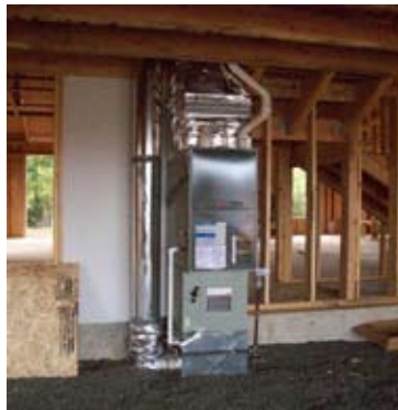
Tour Home with Energy Star System
