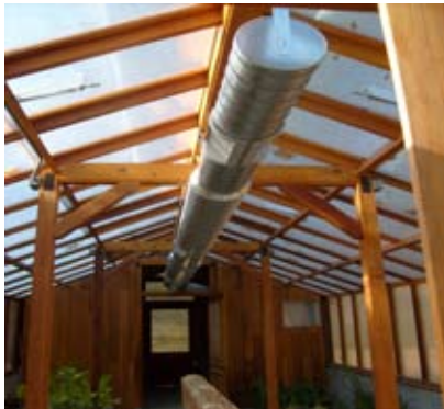
Custom Ductwork in a Green House
